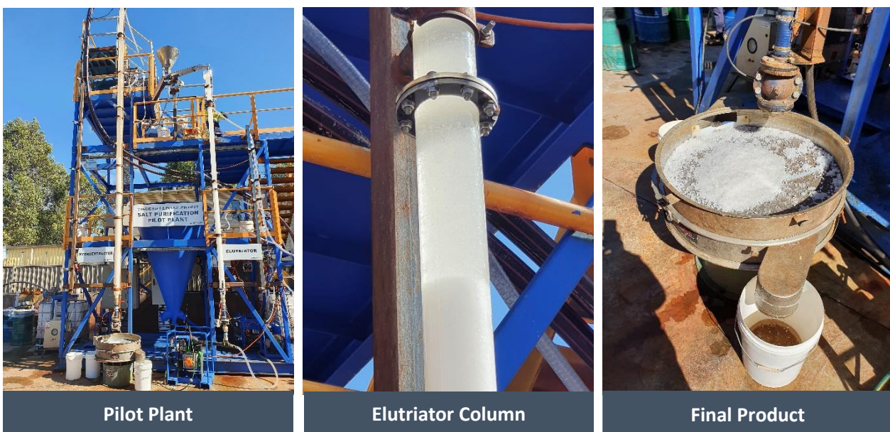
Figure 4: Salt Pilot Plant
