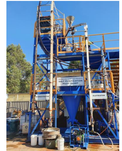
SALT PILOT PLANT (PERTH)
