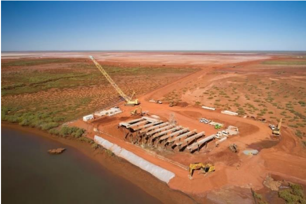
Figure 1: Seawater Intake Station and Pond 0
