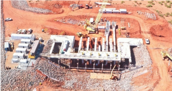
Figure 1: Seawater Intake Station
