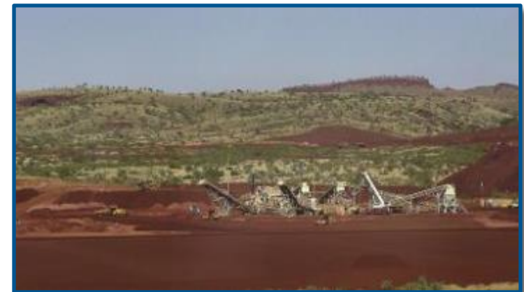
Iron Valley Commissioning – August 2014
