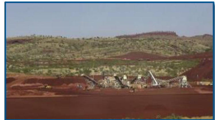
Iron Valley Commissioning – August 2014
