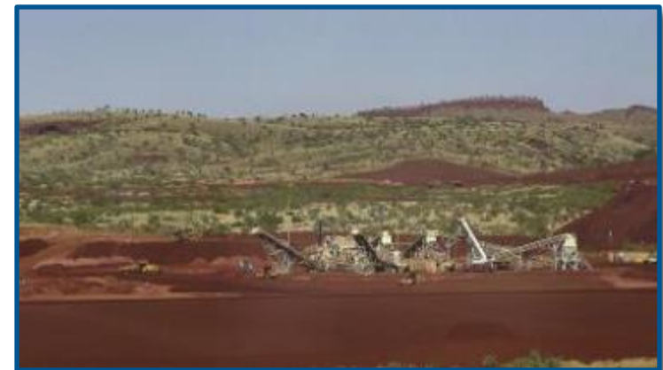
Iron Valley Commissioning – August 2014
