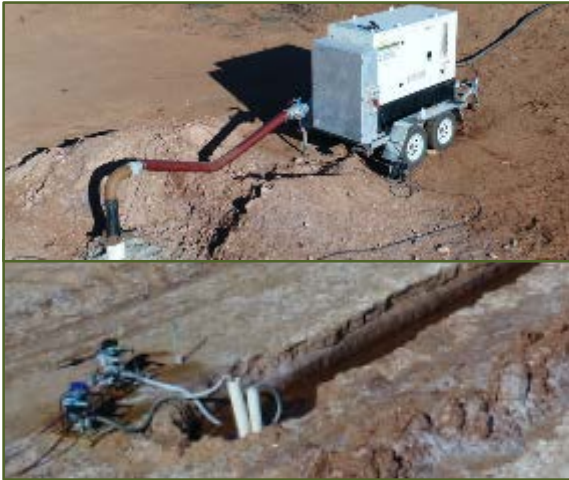
Brine Pumping from Bores and Trenches >160 Million litres successfully pumped to date
