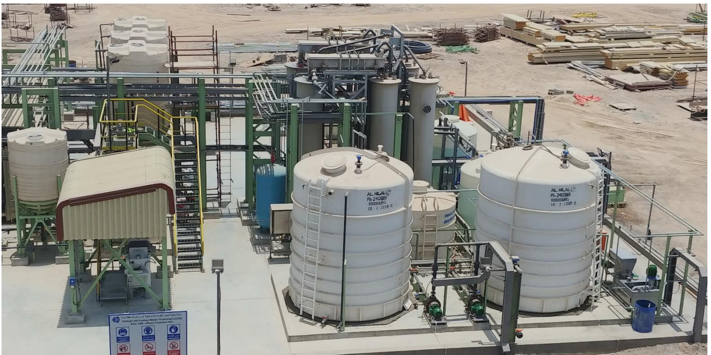
Figure 4 - Clean TeQ's water treatment solution installed within the effluent treatment plant on site in Oman
