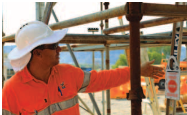
Luke Masterson, Health and Safety Advisor, undertaking a safety audit on scaffolding as part of ERA's Critical Control Monitoring Plan.
