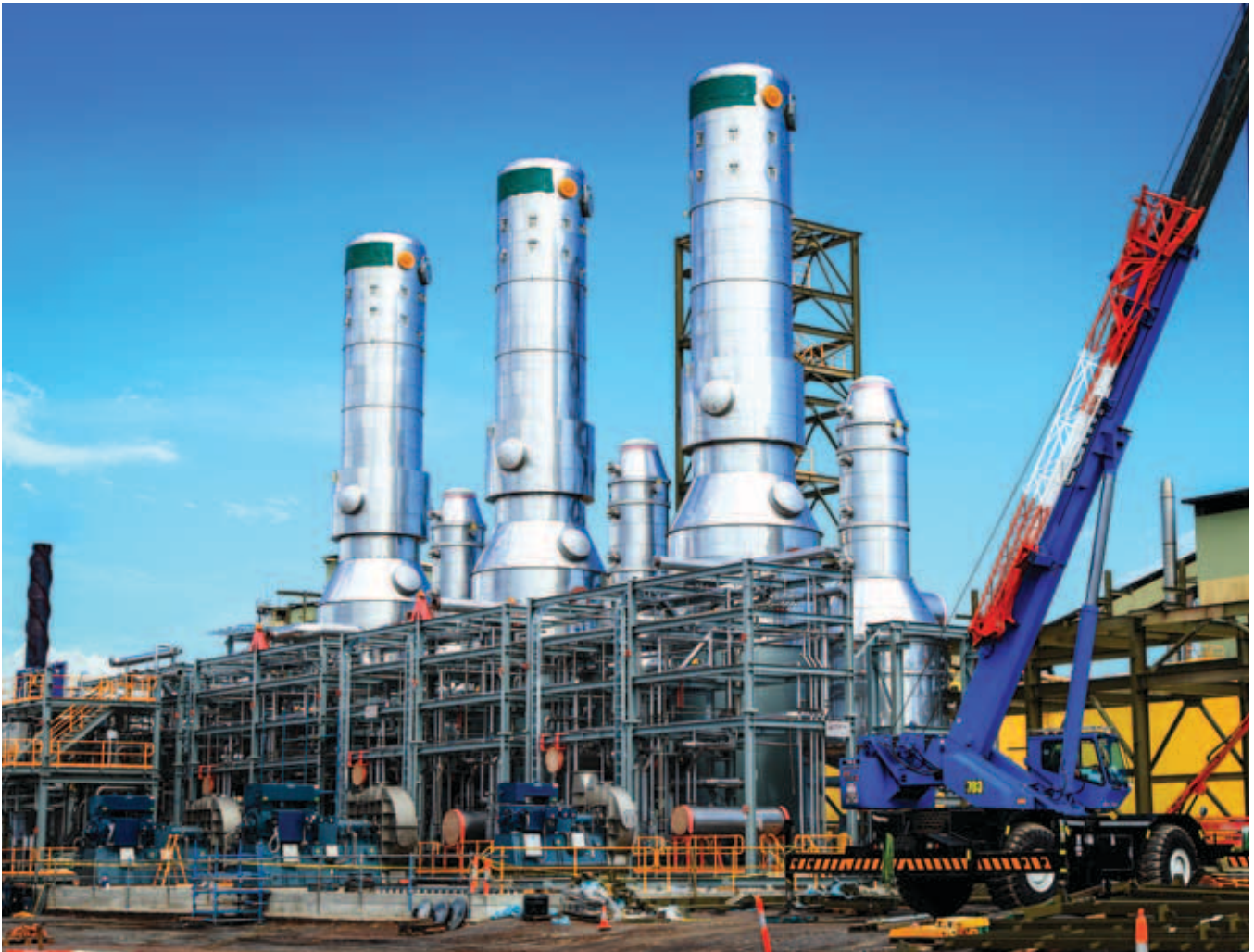
The Brine Concentrator project is on schedule and on budget and is due for commissioning in Q3 2013.
