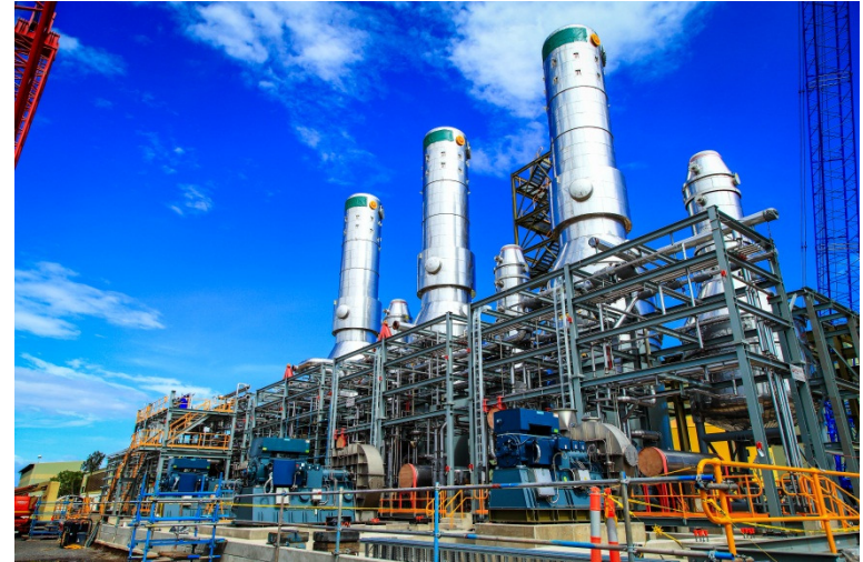
The Brine Concentrator is expected to be commissioned in Q3 2013
