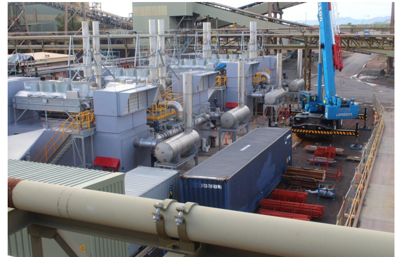
Brine Concentrator Power Station
