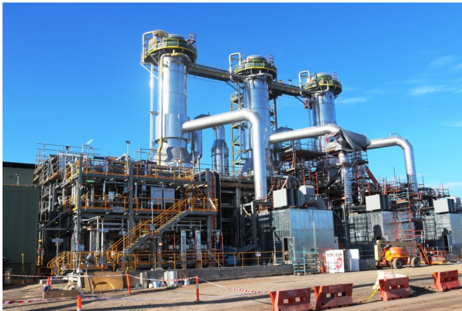
The Brine Concentrator expected to be commissioned in Q3 2013
