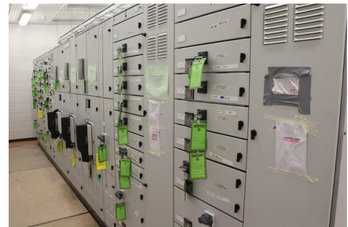
Power substation undergoing testing ready for commissioning
