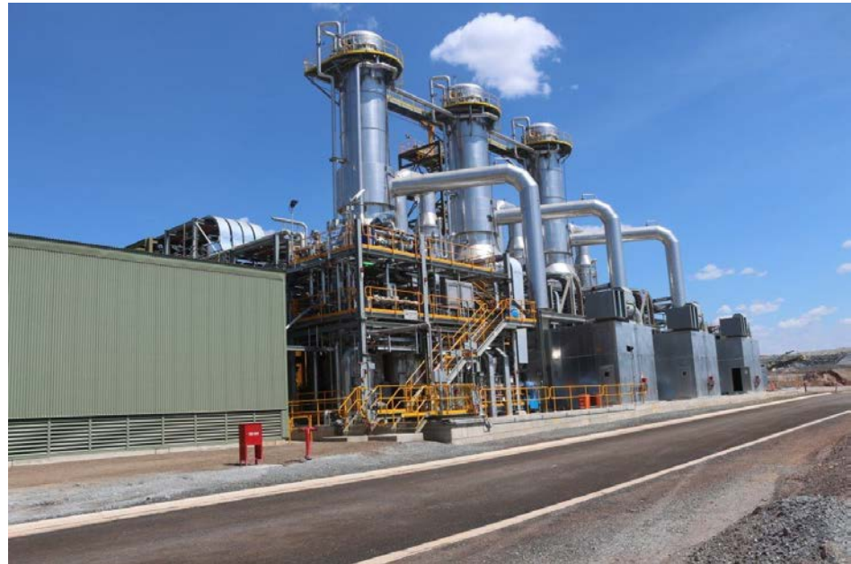
The Brine Concentrator is commissioned
