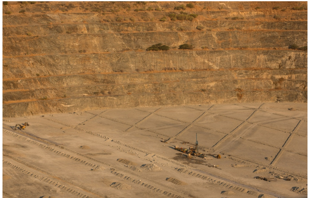
Drainage installation in Pit 3 to prepare it for final storage of tailings, December 2014
