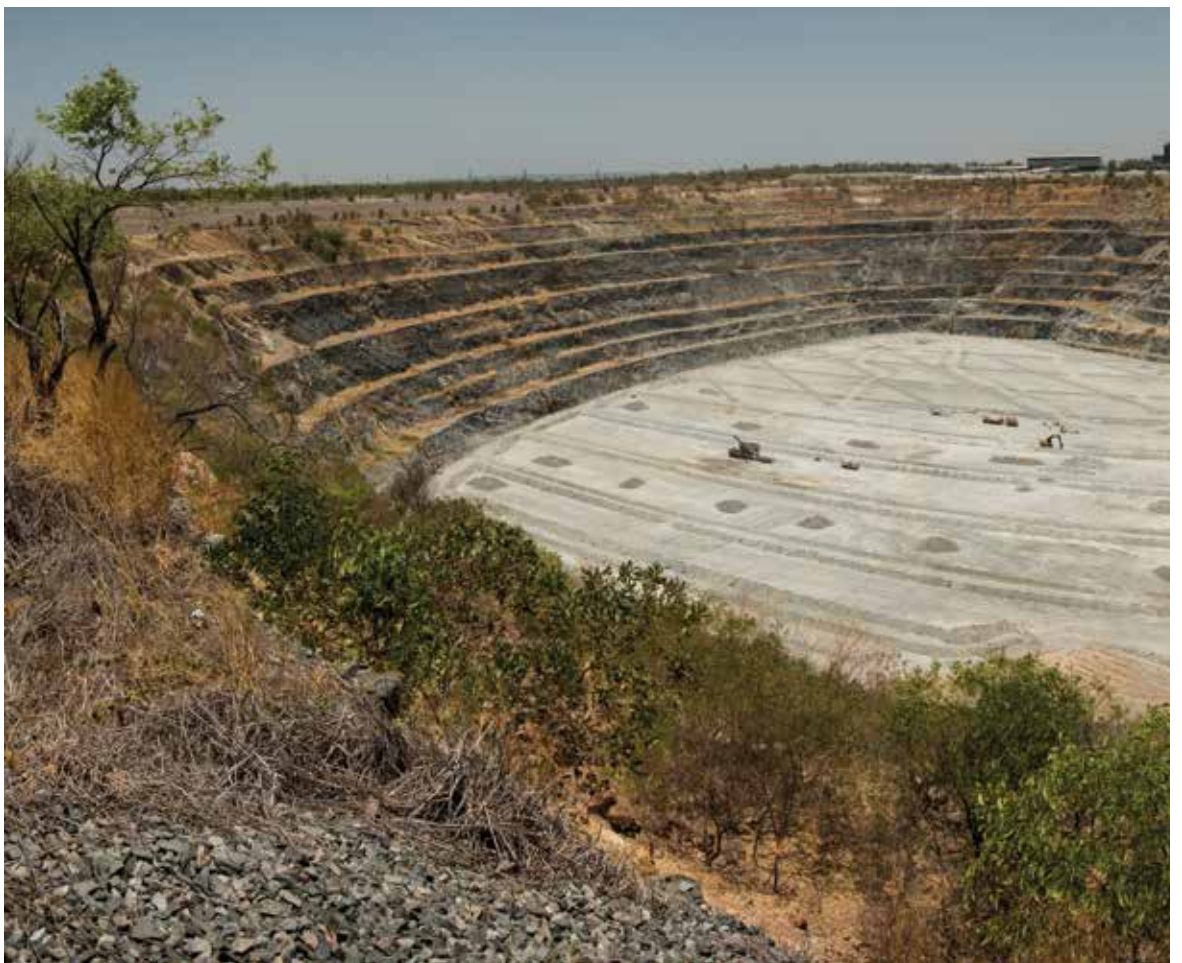
► Installation of the drainage system in Pit 3, December 2014, to convert the pit to receive tailings as part of Tailings and Brine Management program
