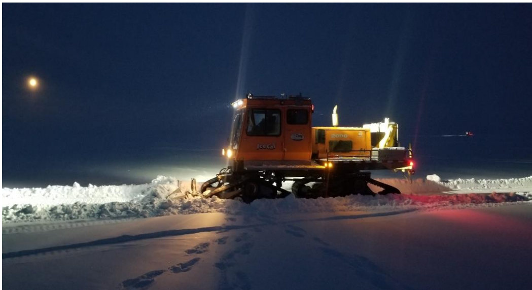
Figure 1 | Ice road construction commences in preparation for mobilising the drill rig to the Winx-1 well location
