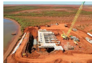
SEAWATER INTAKE STATION
