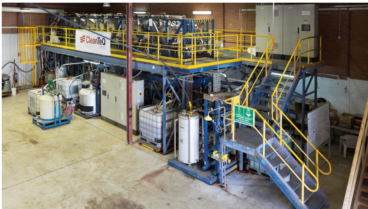
Clean TeQ's proprietary Resin-In-Pulp (cRIP) process demonstration plant
