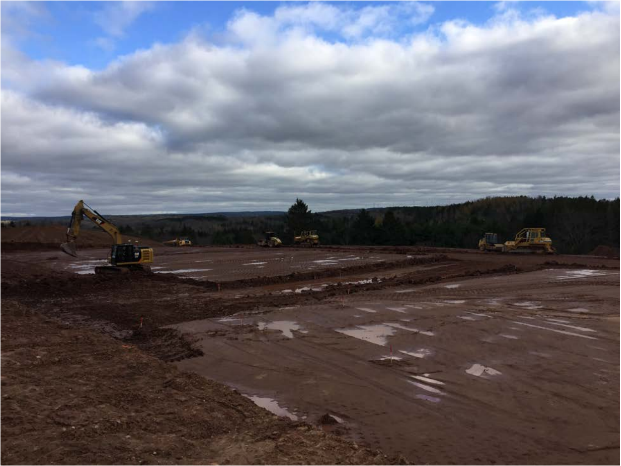
Picture of construction commenced at Creso's Mernova Medical facility, Nova Scotia, Canada.
