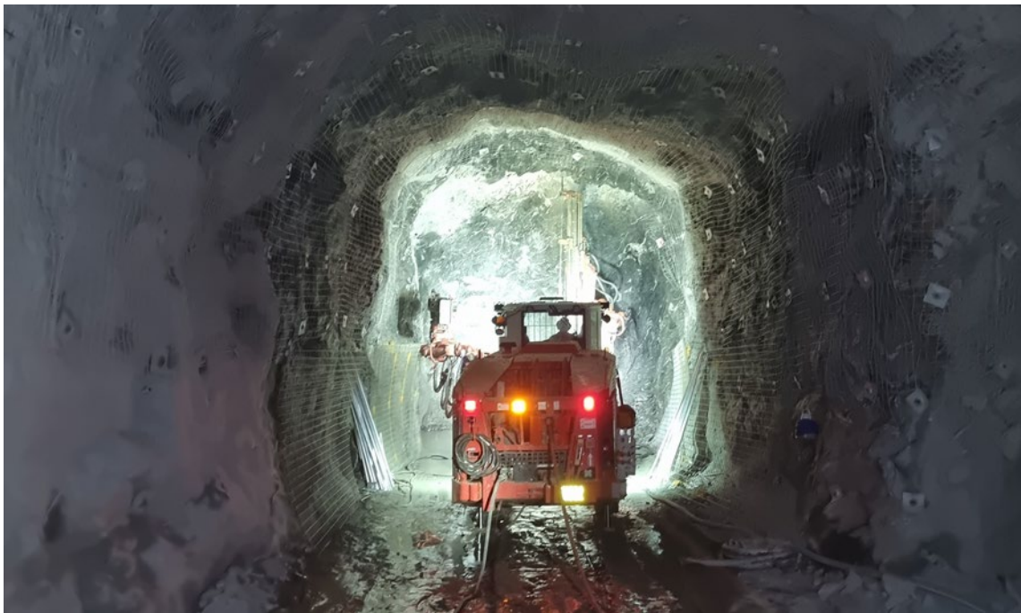
Figure 2 – Work has commenced on the decline to access the Avoca Tank orebody.
