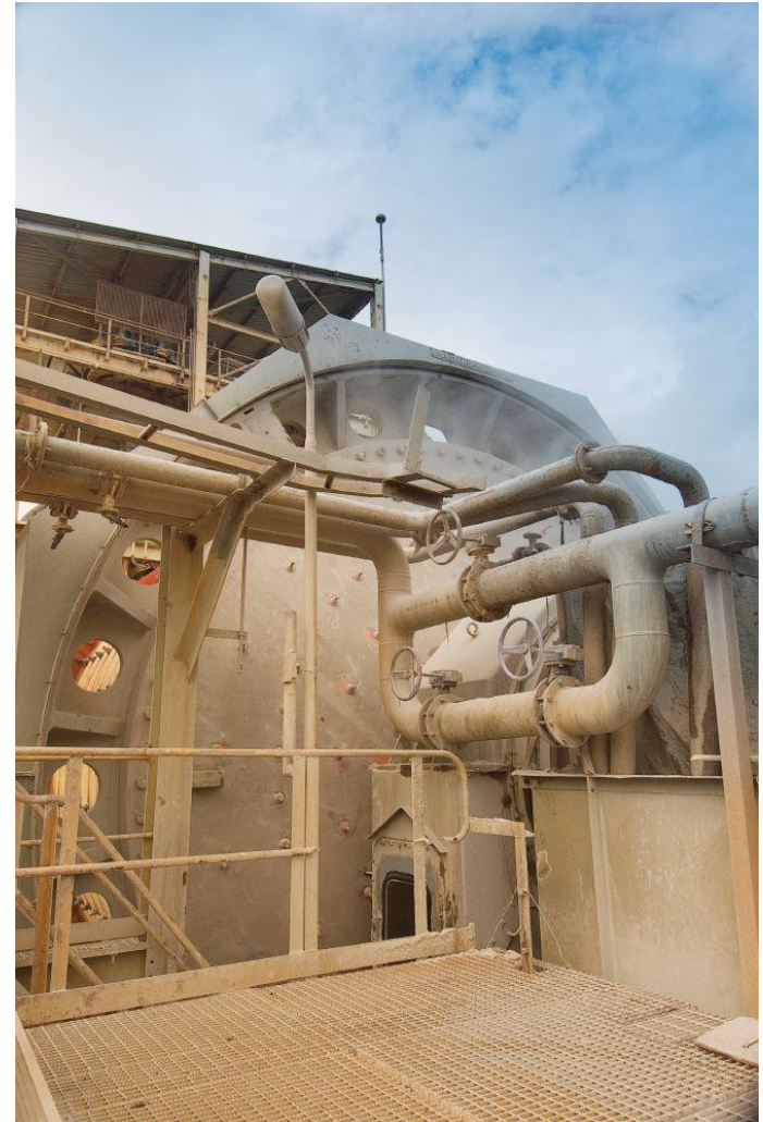
3.5 MW Semi Autogenous Grinding Mill
