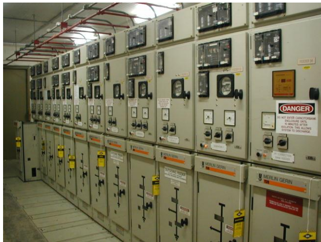
Network distribution and control
