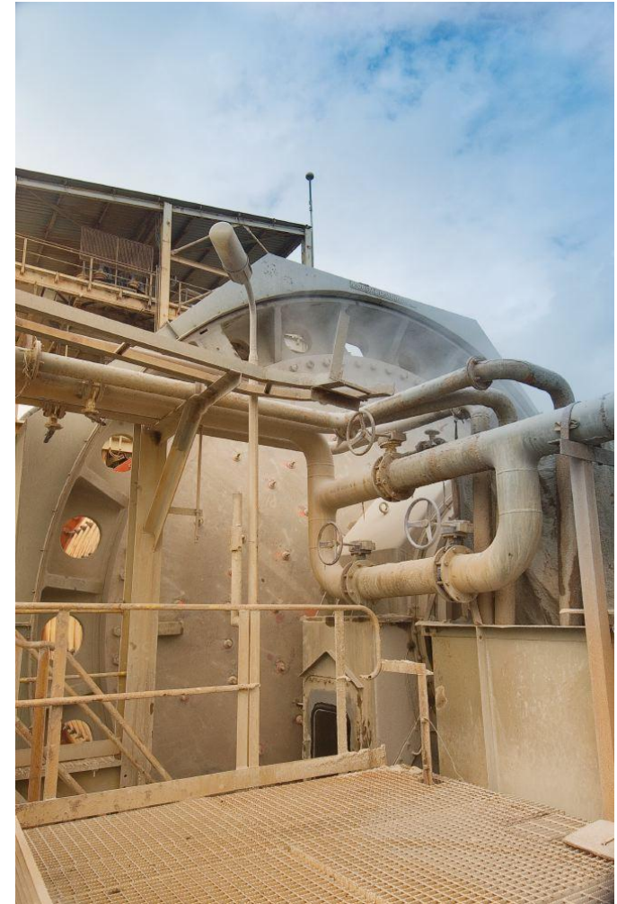
Single stage 3.5 MW SAG Mill.
