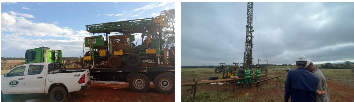
Figure 2 - Rig mobilisation (left) and diamond drilling operations (right) supporting the expanded Piracanjuba field programme. Photographs provide operational context only and do not report Exploration Results.
