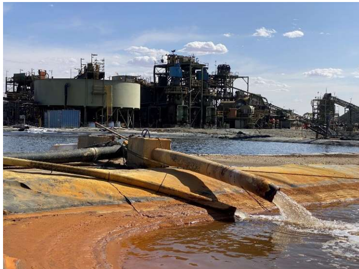
Fresh water being delivered to Tritton Processing Plant
