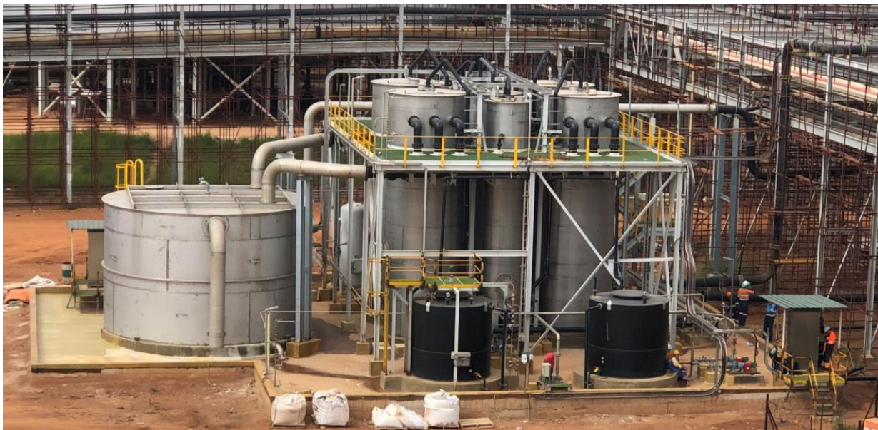
Figure 5 – Clean TeQ Continuous Resin-In-Column Ion Exchange plant in DRC
