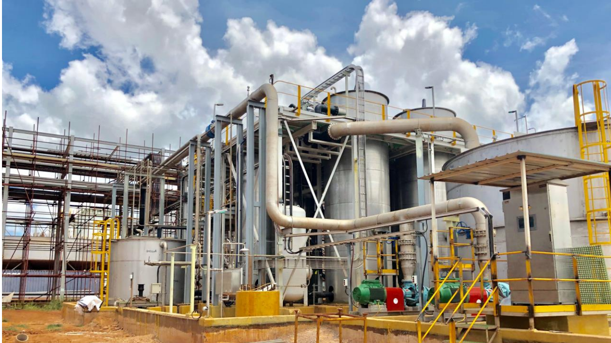
Figure 6 – Clean TeQ Continuous Resin-In-Column Ion Exchange plant in DRC
