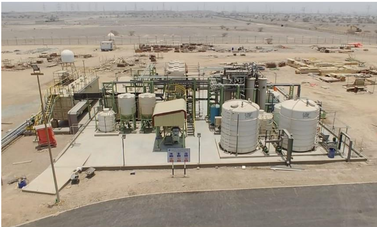
Figure 4 – Clean TeQ CIF® plant constructed and awaiting commissioning in Oman
