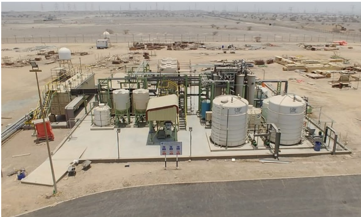
Clean TeQ's proprietary DESALX® (two-stage CIF®) plant in Oman
