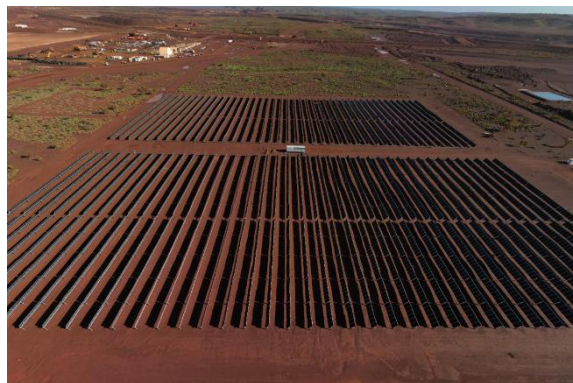
Solar array at Ken's Bore
