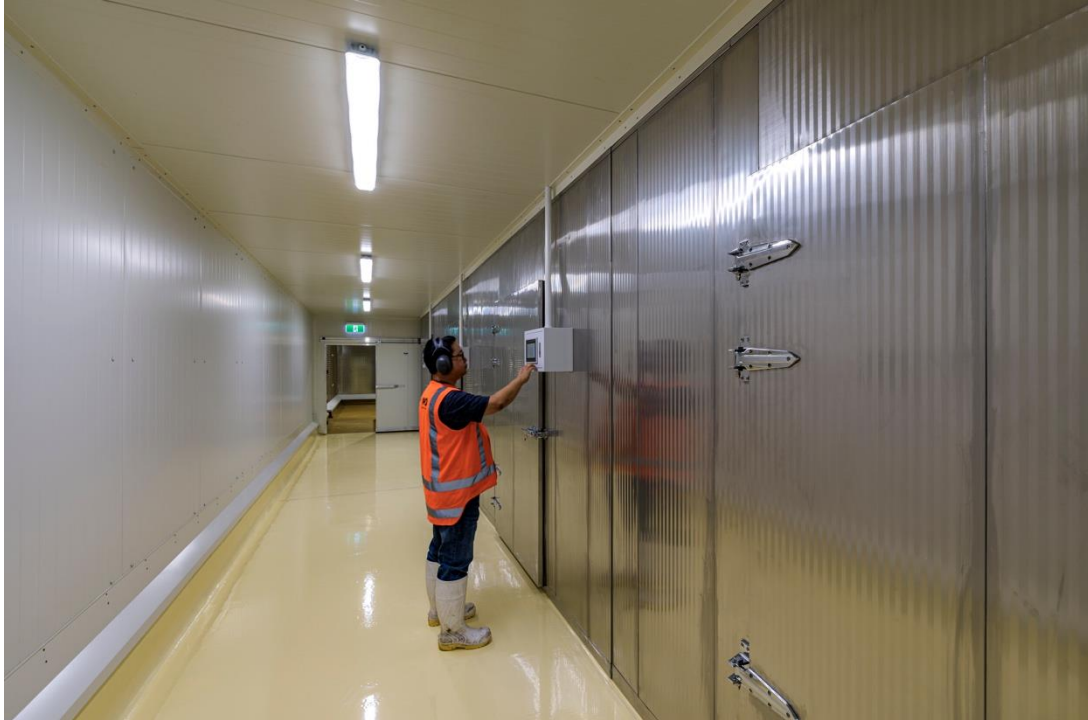
Image 2 – Hygiene / Drier Entry Zone - Final Commissioning and Testing
