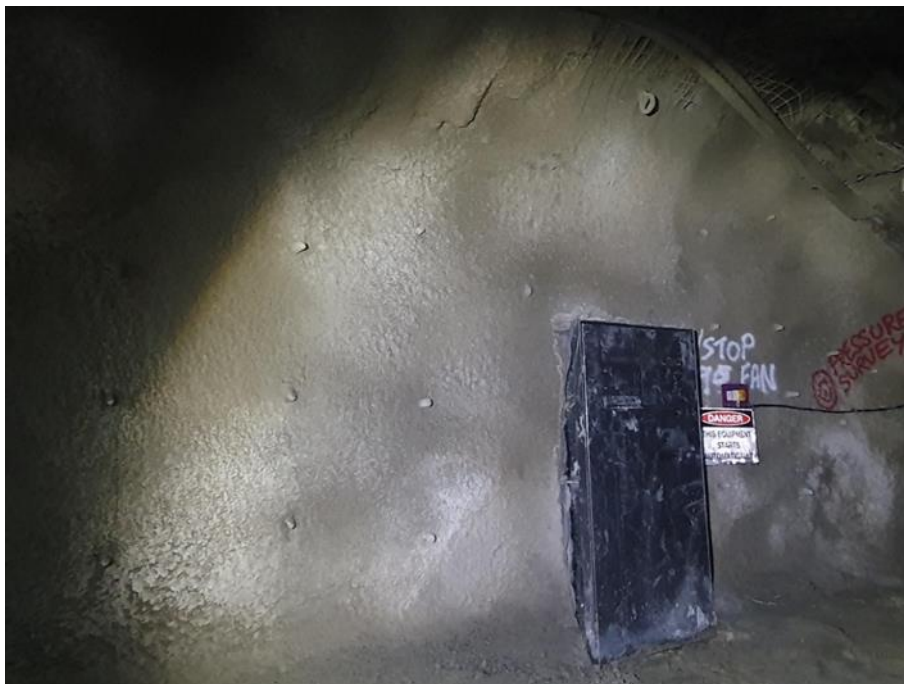
Figure 5: Vent door closing off ventilation recirculation, set in shotcrete and cable bolts for additional ground support.
