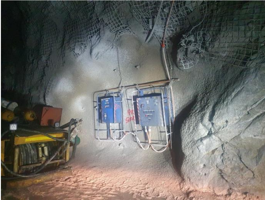
Figure 6: New electrical substations to distribute high voltage power.
