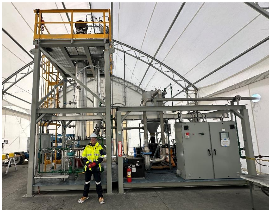
Hazer COO Tom Coolican at the FortisBC pilot rig.
